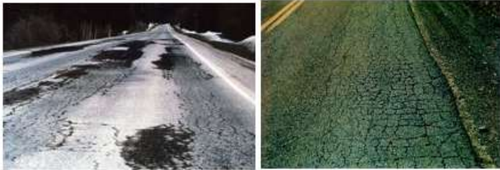
Figure 4. Images of Fatigue Cracking in Asphalt Pavement (Pavement Interactive, 2009)
