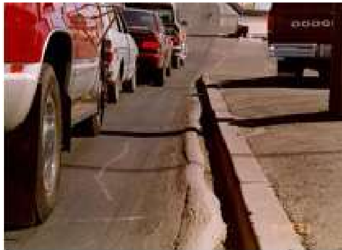
Figure 2. Rutting on side curb of Asphalt Pavement (Pavement Interactive, 2009)
